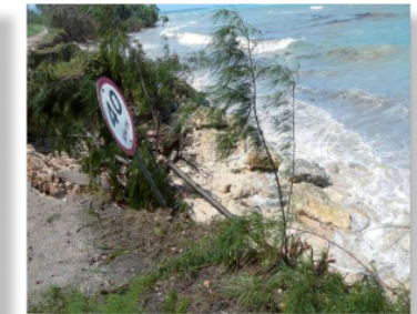
Destruction of coastal road and tree during Tropical Cyclone Rene, 2010, SNC Project Tonga, 2010
