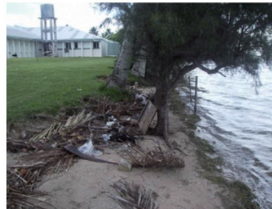
The hospital fence in the sea, Lifuka, Ha'apai, NEMO, MOW, 2009
